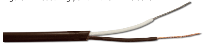
Figure 3: Cable end at the measuring channel
