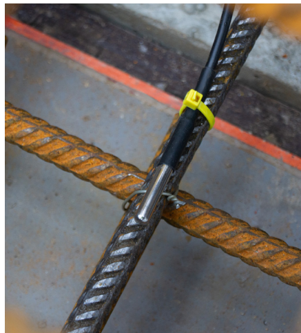
Figure 2: Digital Thermocouple mounted
