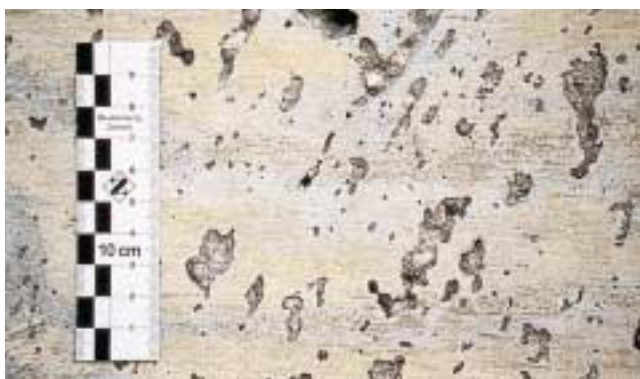
Fig. 3: Pore formation in a fair-face concrete surface.
