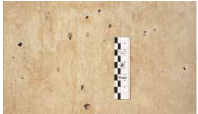
Fig. 4: Pore formation in a fair-face concrete surface.
